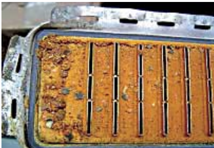
Deposits caused by oil leaking
